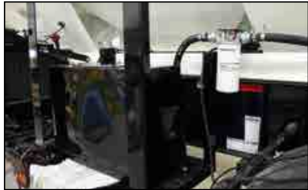
Fig 72 - Hydraulic reservoir and filter
