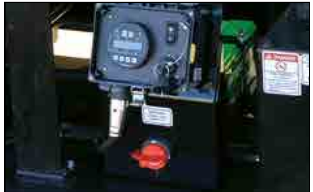
Fig 40 - Engine control and battery lock-out
