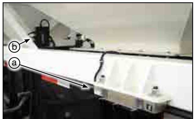
Fig 18 - (a) Load Cell, (b) weigh scale junction box
